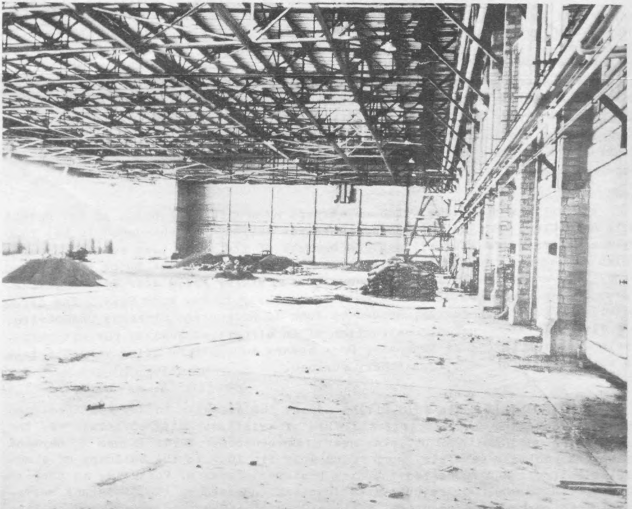
A corner of the huge hangar being built for the City by the WPA
